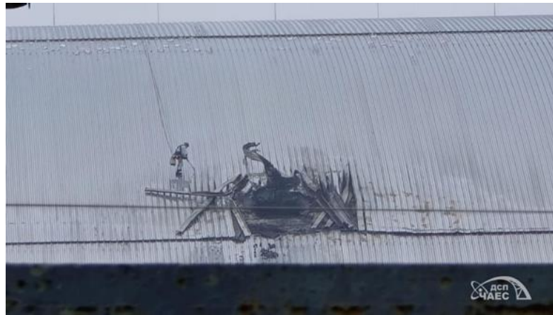
Fig. 1. Structural damage to the roof of Unit 4 of the Chernobyl Nuclear Power Plant following a missile strike.
